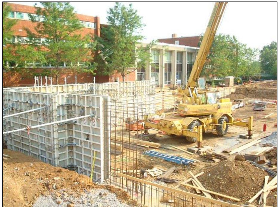
EdR oversees all construction work, such as the first phase of the on-campus housing revitalization at the University of Kentucky
